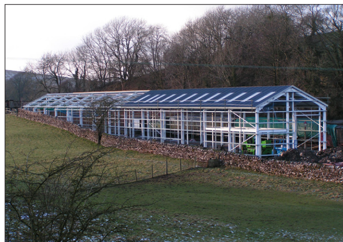
Below: The framework for the new shed and workshop under construction. The structure is now externally complete and the track is in situ, with the concrete floor sections now in the process of being poured. Mike Thompson / Stainmore Railway Co
