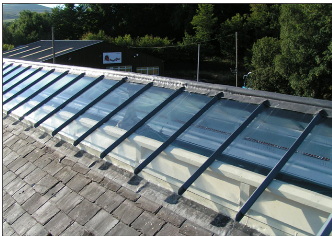
Above: Repairs to the Darlington side trainshed roof have recently been completed, retaining the original glazing and making the structure watertight for the first time in preservation. Mike Thompson/Stainmore Railway Co
