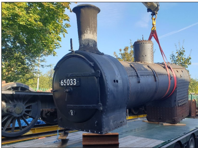
Above: The boiler of J21 No. 65033 is lifted from its frames for the first time in over four decades at Locomotive Maintenance Services, ready for stripping and assessment to begin. LMS/LCLT
