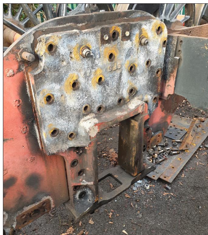
Below: The need for new frames is obvious when reviewing this picture showing the condition around one of the horn guides! LMS/LCLT
