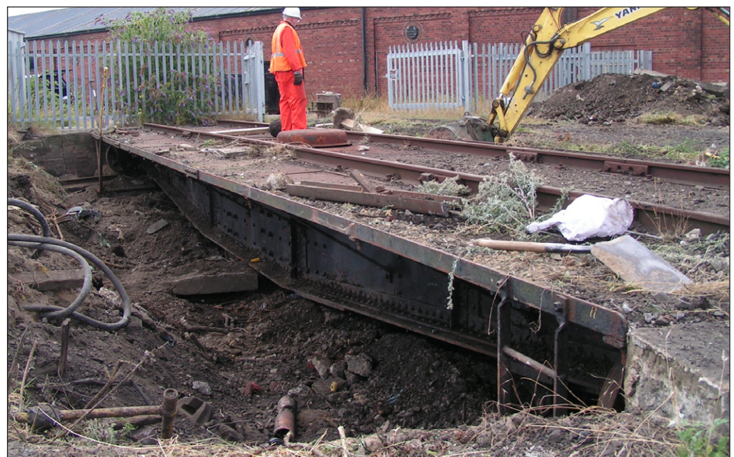
Right: The remarkably complete replacement 50ft turntable obtained for Kirkby Stephen East, pictured during its extraction. Mike Thompson/Stainmore Railway Co
